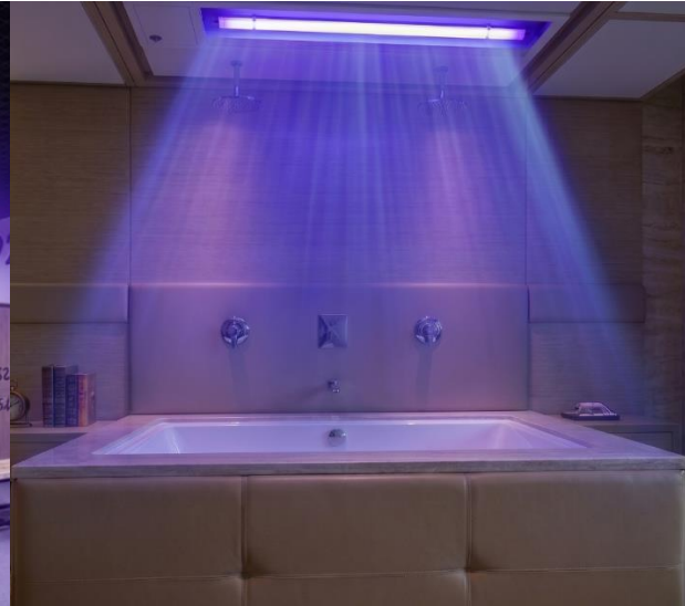
Locker room: UVC active in unoccupied mode, instantly switches to LED when guests enter.
